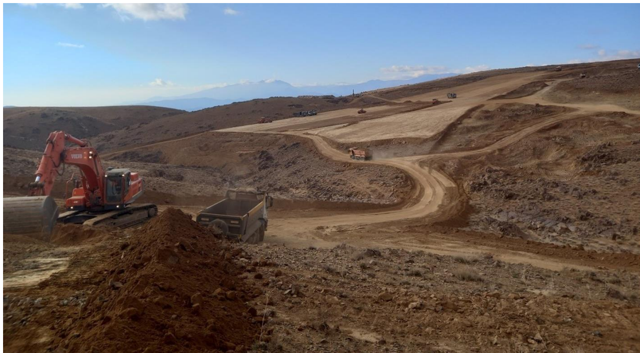
Figure 4 – Start of construction of tailings storage facility for the new Zgounder processing plant.
