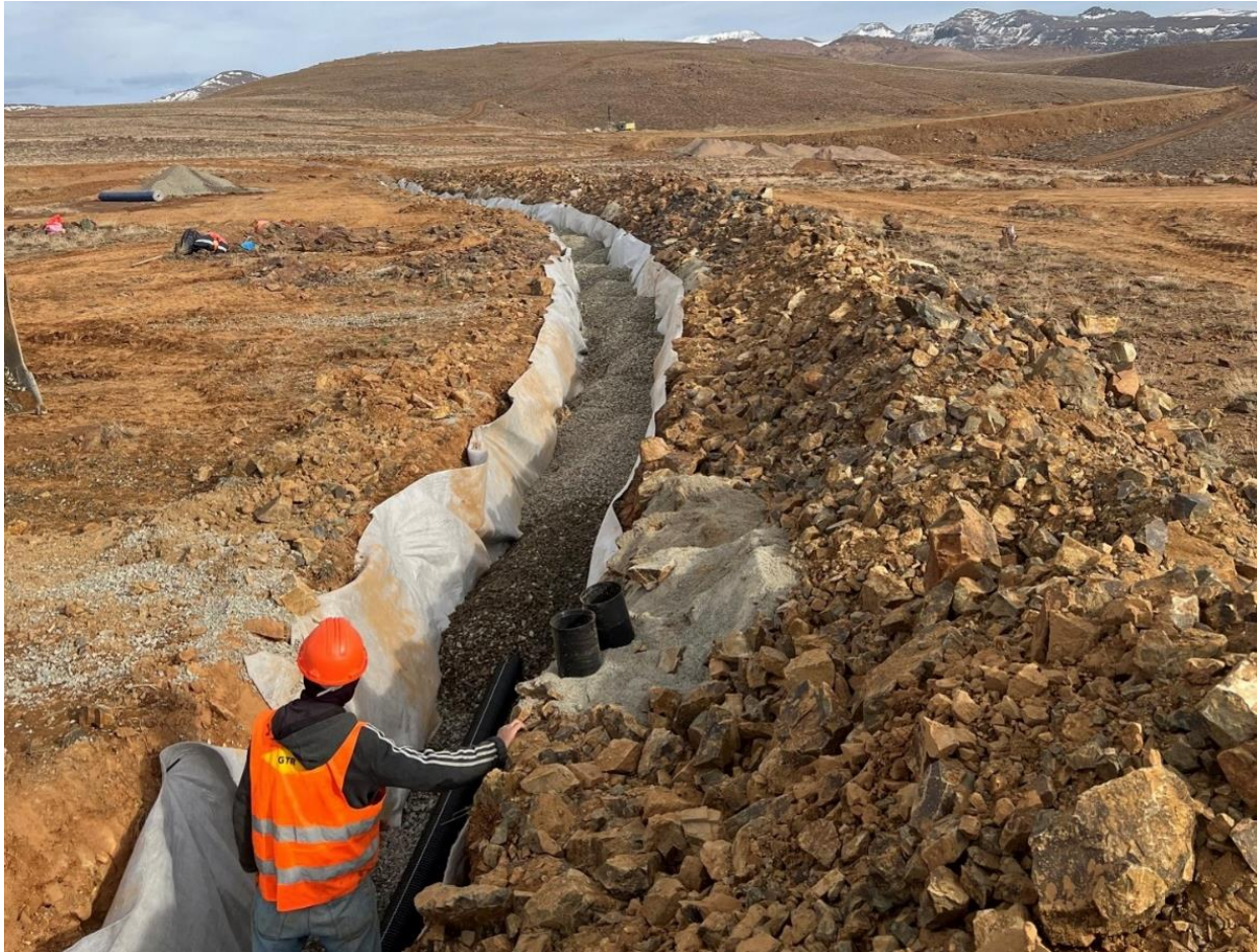
Figure 5 – Installing the drainage system at one of Zgounder’s new water storage basins
