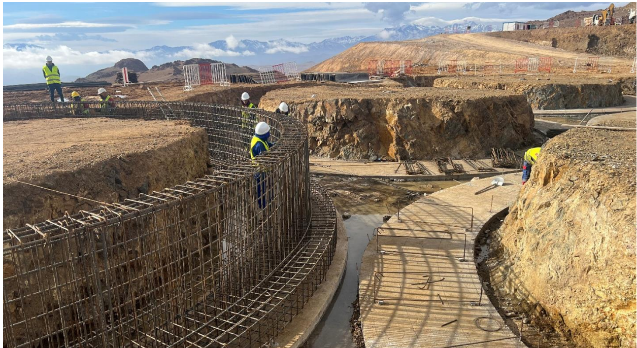
Figure 4 – Erecting structural steelwork for the leach tanks at the new Zgounder processing plant
